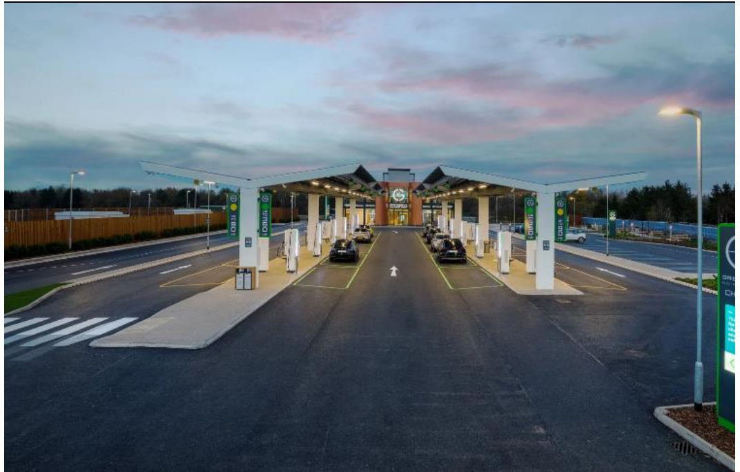
Figure 4.5 Example of a safe fast public charging station
